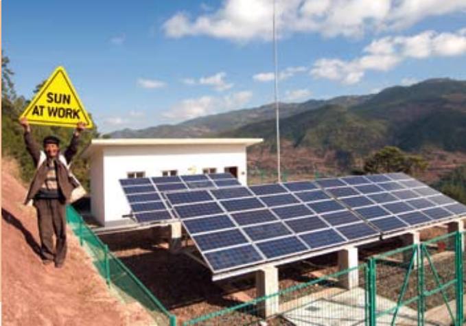
Rural electrification of off-grid regions
